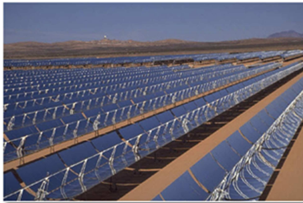
Figure 1 - Typical parabolic-trough solar field
